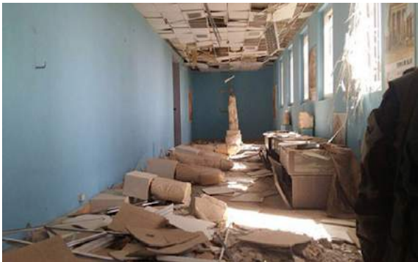
Figure 63. Damage inside gallery (posted by DGAM; March 28, 2016)
